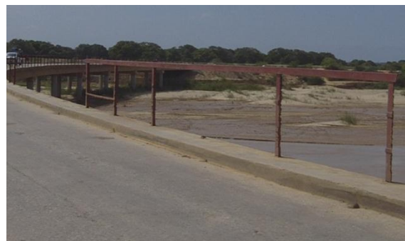
Photo 11 Insuffisance de garde-corps
