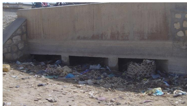
Photo 7 Dalot obstrué PK 2+040
