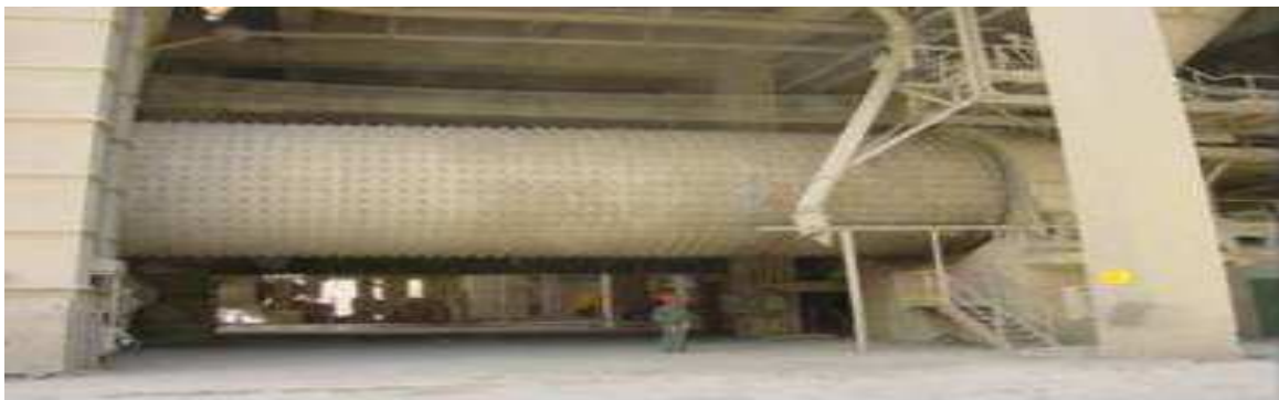
Figure 16 : broyeur (broyage cuit)
