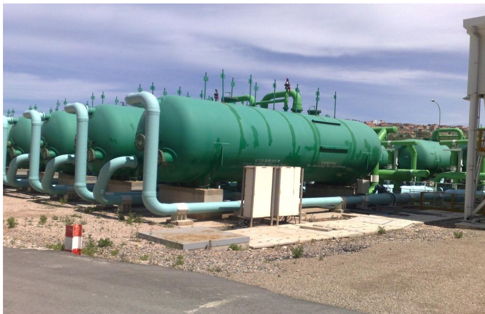
Figure III.9: photo des filtres multicouches
