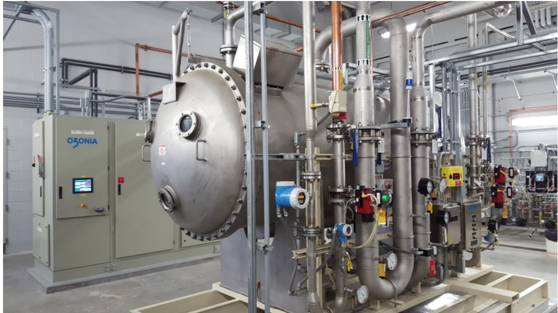
Figure 6.4 A 400kW ozone generator and its PSU in the background, where we can see in the foreground the process piping, valves, and various meters used to control the gas and the cooling water flowing into the generator vessel
