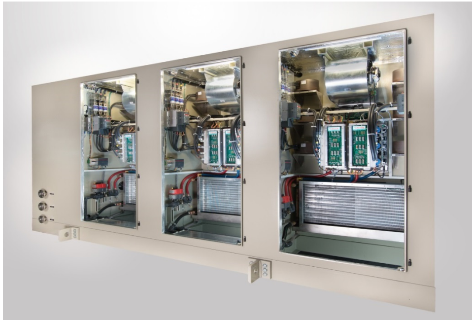
Figure 6.11 A 1.2MW ozone generator I-PSU™, doors removed for clarity
