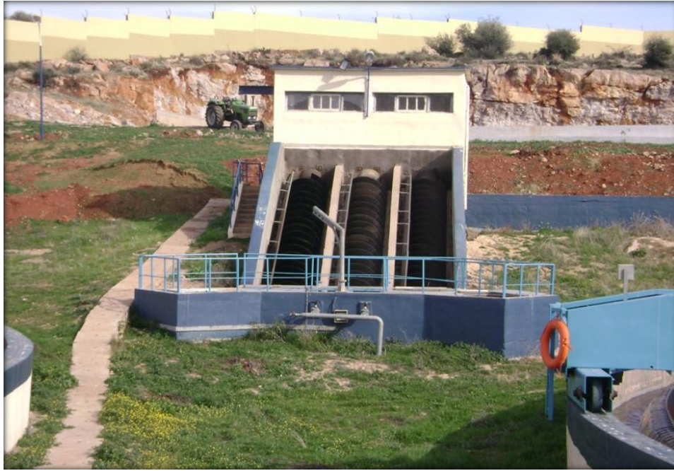
Figure III.11: Photo des vis d'Archimède [31]
