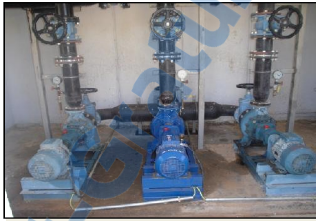
Figure III.11: Le Poste de Recirculation (14/05/2012)
