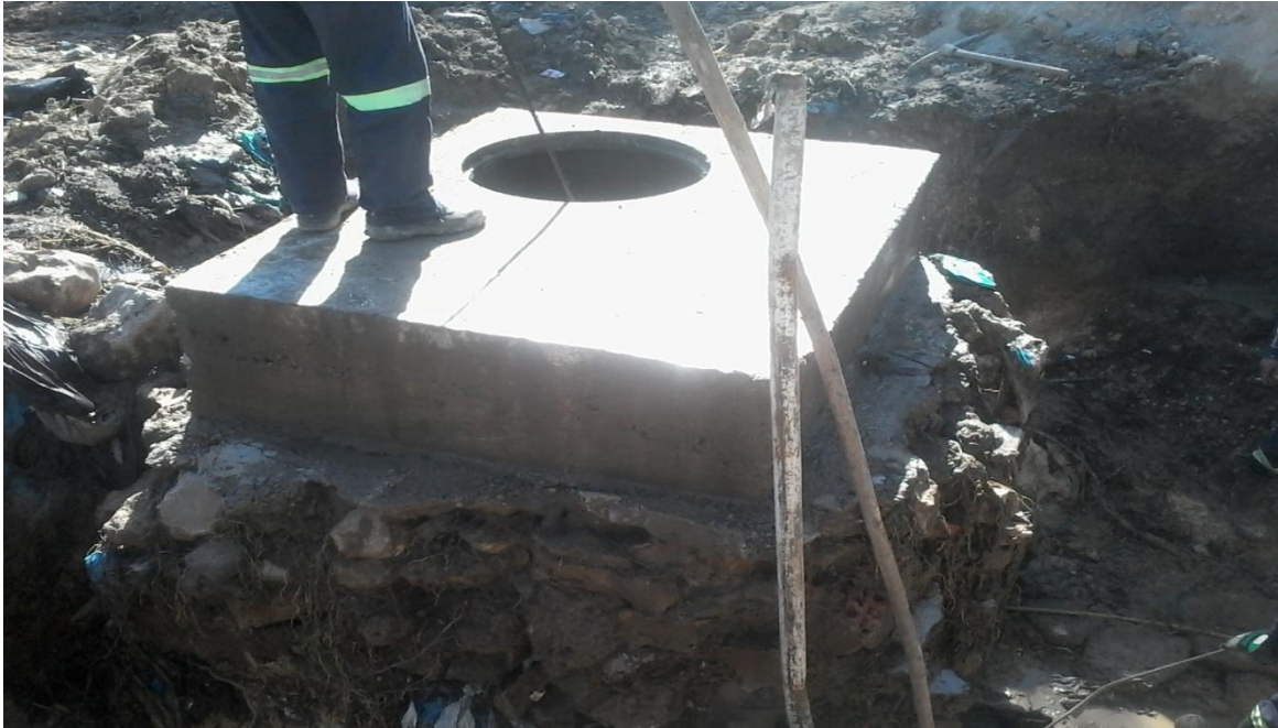
Figure. II. 19 : Regard de visite [16]
