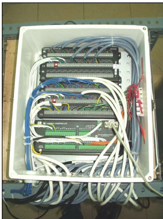
Figure 6 : Centrale d'acquisition Campbell CR10X
