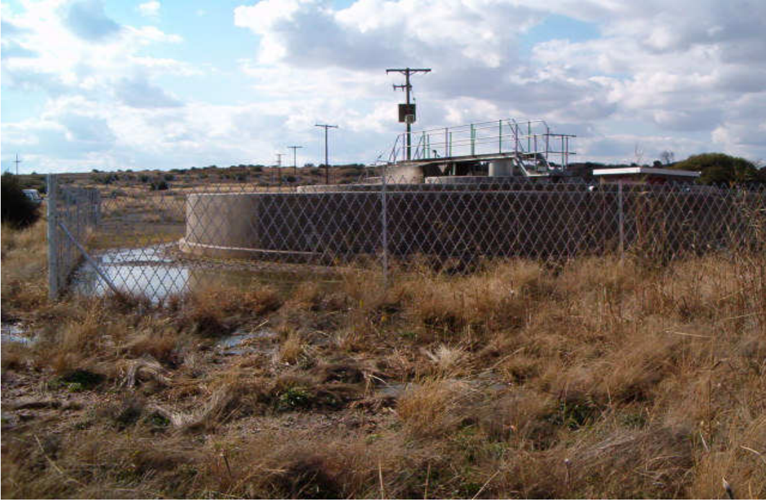
Figure 4-2. A sewage treatment package plant constructed in 2002 that two years later no longer functioned optimally as indicated by the ponding of effluent on site.
