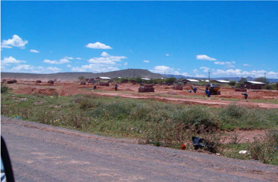
Figure 2-2. A low-income housing development being constructed in the Tsolwana municipal area of the study area 1 .
