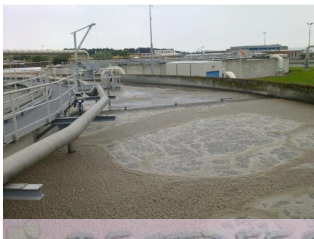
Figure 6.2. Activated sludge in BNR reactors at Mangere Wastewater Treatment Plant, New Zealand
