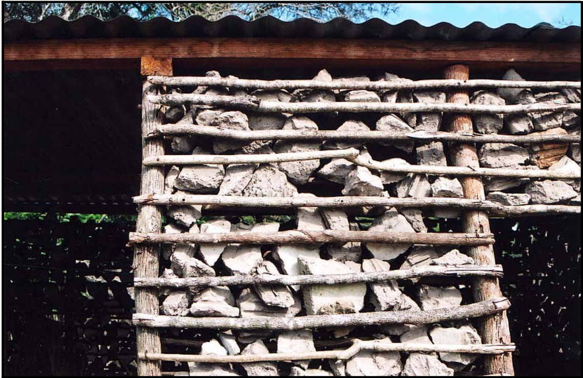
Figure 9: A rectangular single room house in construction. This picture illustrates the packed stones within a wooden frame wall structure, a new building method observed in the Manqakulane community. The roof structure is also clearly seen and shows the corrugated iron plates resting on a minimalist plank frame. Photo by J. Gaugris: Manqakulane community, northern Maputaland, KwaZulu-Natal, South Africa, 2002.
