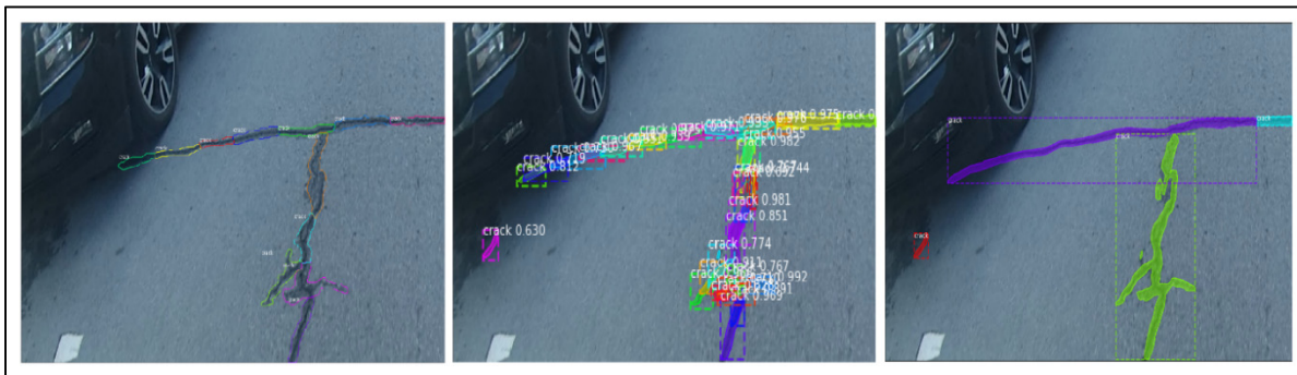
Figure 3.43 From left to right: RGB image with the GT; crack segmentation before applying the merge function; and after applying the merge function
