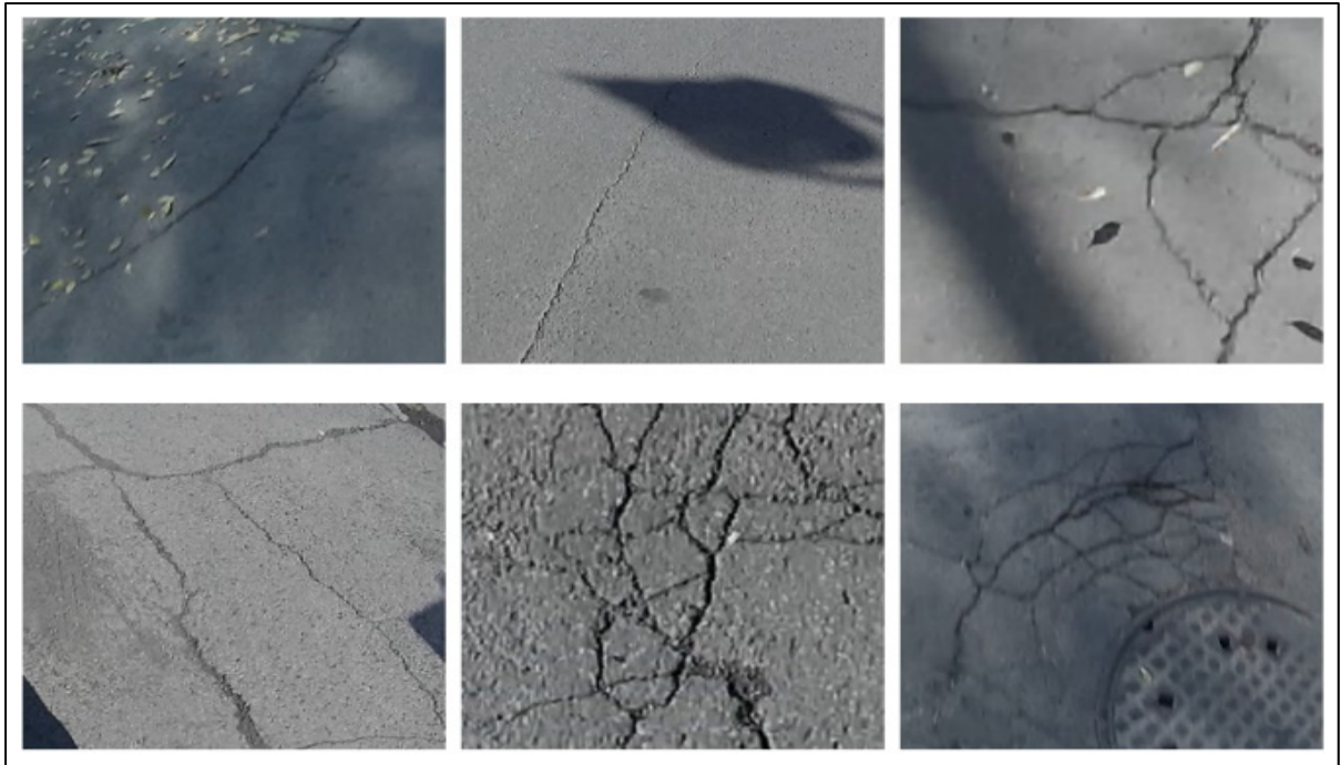
Figure 3.40 Cracks in different lighting conditions, with random objects and different pavement materials
