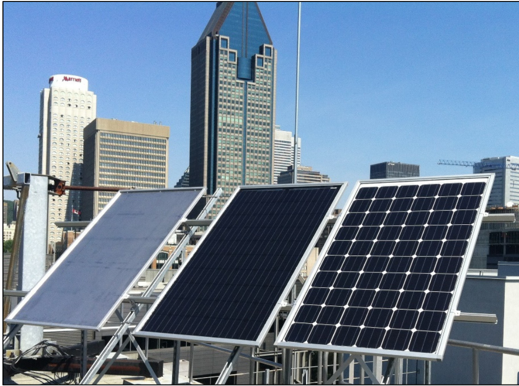
Figure 2.7 The three solar absorber plates installed in the experimental setup
