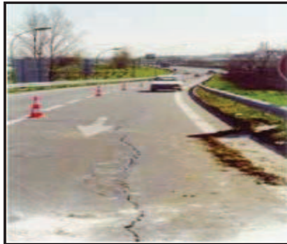
Figure 2.11 Fissuration due au retrait-gonflement (Ferber V., 2005)
