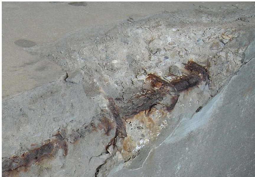
Figure II.1 Pathologie due à la carbonatation [1].
